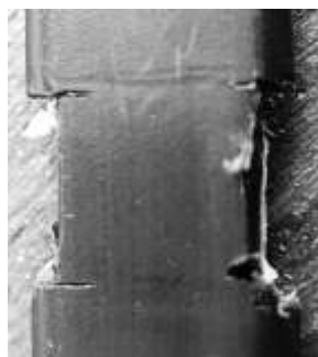
Removal of insulation at points B to C and J to K on both sides of the twin lead
