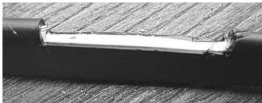
The cut out gap opening with one inch of conductor removed. See points D and E on the sketch.
